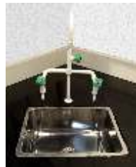
Laboratory Sink with Utilities
